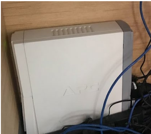
Circulation Desk UPS (Battery Backup)
