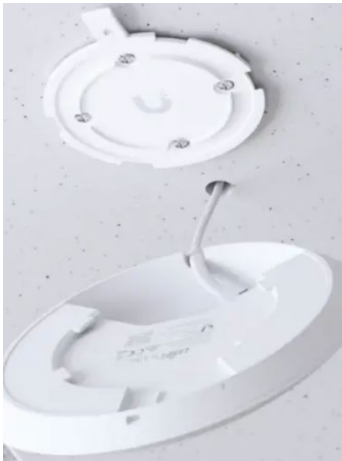
Crestron WIFI Access Point in the West Meeting Room Ceiling
